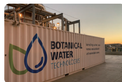
Water Harvesting Unit (WHU)
